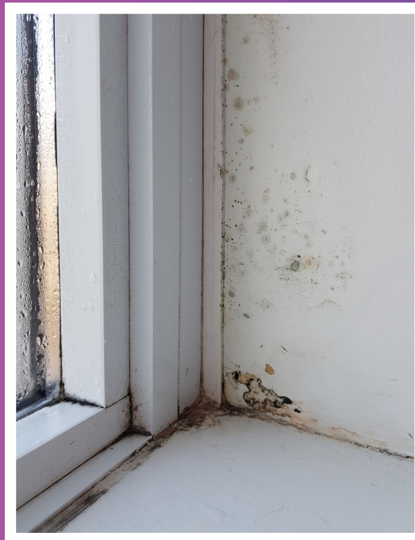
Example: Condensation and mould build-up on a window frame caused by excess moisture and poor ventilation.
